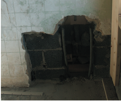
The interior walls were 12 inches of plaster and concrete. "It was built like a bomb shelter," said Estes.
